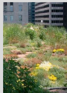
Intensive Green Roof - Much thicker build up but can accommodate a wider variety of plant species
