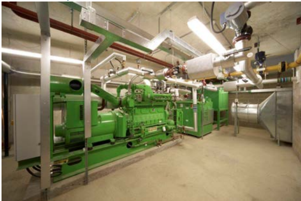
Figure 18: CHP engine at Grosvenor Waterside, SW1
